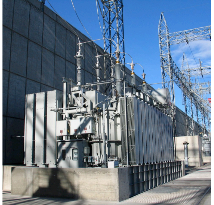
Fig. 4 Application of FO sensor for cooling control on a 240 MVA transformer at GCPUD.
